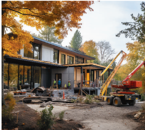
Construction of a modern home in Hawley, Pennsylvania. This passive house utilizes geothermal heating and cooling, solar and batteries for electric generation, and atmospheric water generator to be truly off-grid.
